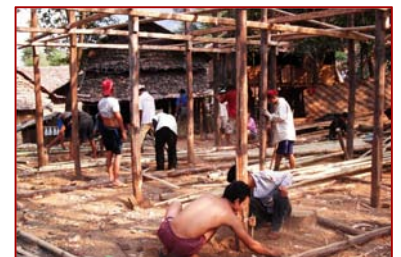
(Below): The construction of a new dormitory at Ler Doh in August benefited from the help of many community members.
